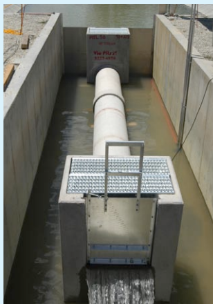
Figure 3: “Unearthed” Murrumbidgee Irrigation meter outlet showing the head/discharge drop boxes (sumps) with the resultant fully submerged pipe.
