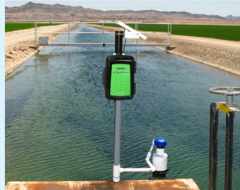
Figure 2: The Series3 MACE FloPro unit installed on Quail Mesa Ranch. An ultrasonic depth sensor (EchoSpan®) is mounted over the crest of the weir.
