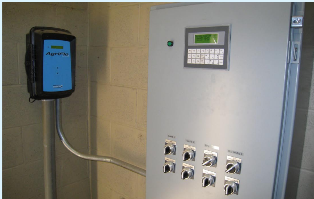
Figure 3: The Series3 MACE AgriFlo unit installed in the control "hut" and interfaced to a Modbus SCADA package that controls the piped off-take
