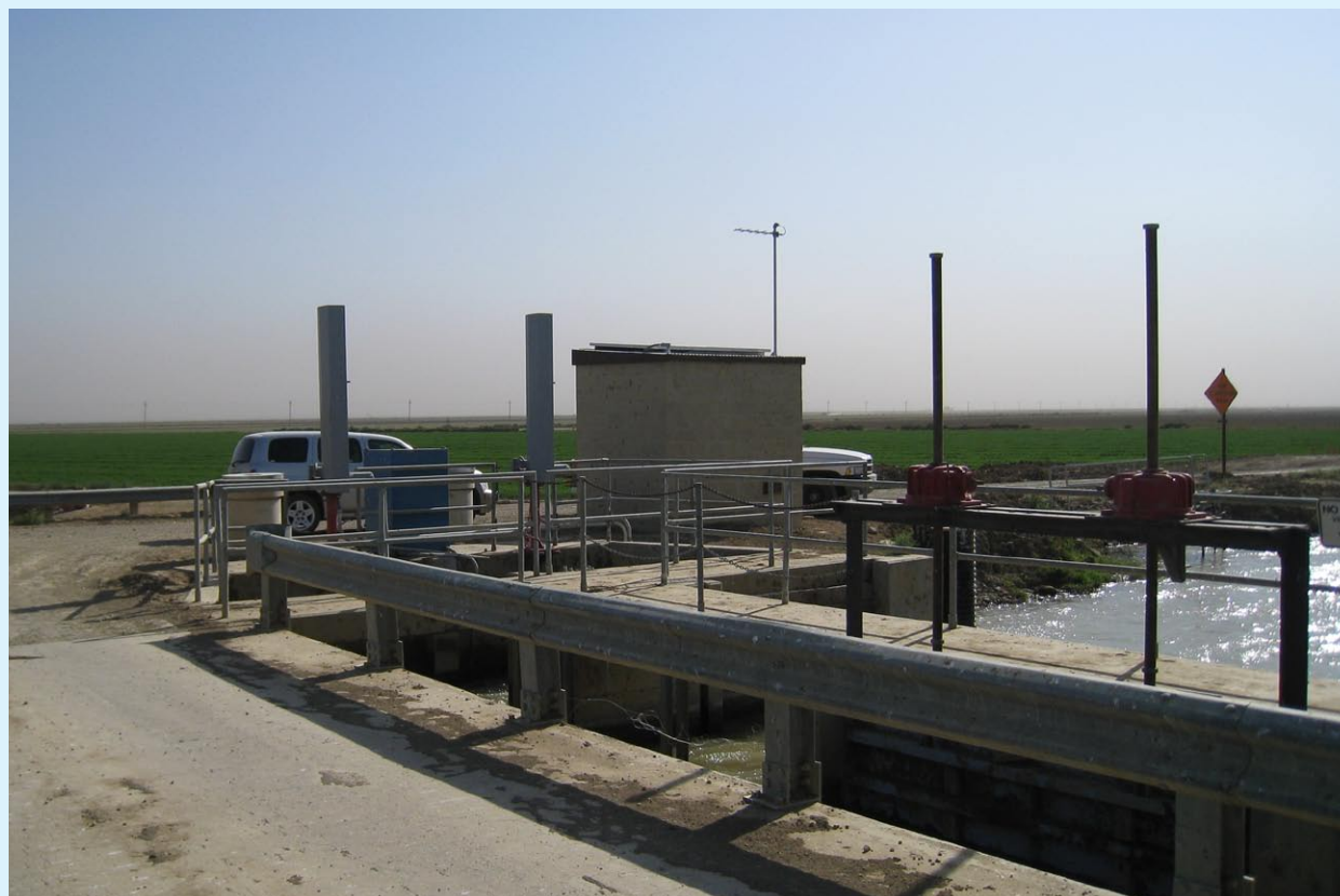
Figure 1: CCID's "O'banion" lateral diversion, near Los Banos, CA, USA.
