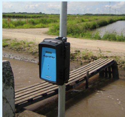
Figure 2: A Series3 AgriFlo installed on the delivery channel of the Costa Rican Tilapia farm.
