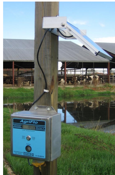
Figure 1: MACE AgriFlo unit installed on a dairy farm in southern Georgia, USA.
