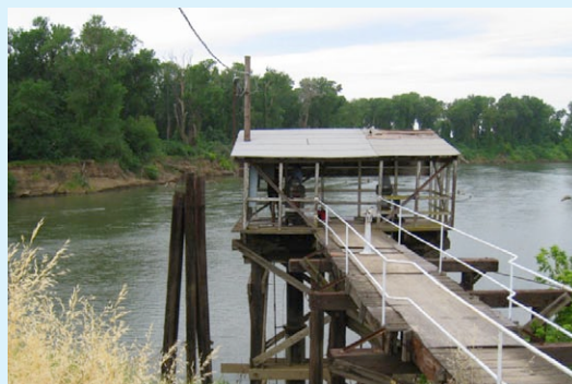
Figure 1: Typical Sacramento River pump-station near Williams, CA with two 18" pumps.
