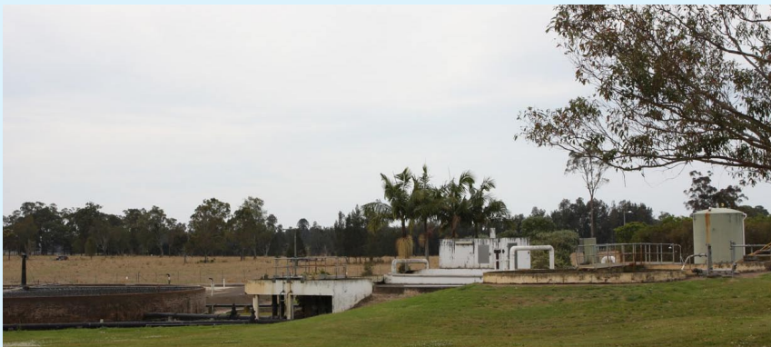
Figure 2: A Typical Mid North Coast sewer treatment plant (STP) near Kempsey, NSW.
