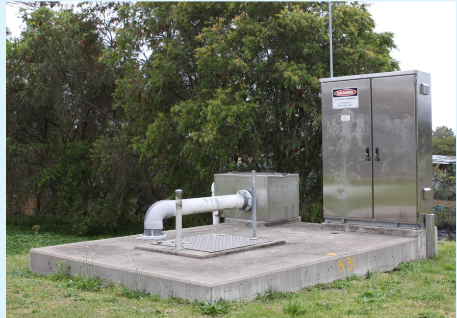
Figure 1: A Typical Mid North Coast lift pump station near Kempsey, NSW.
